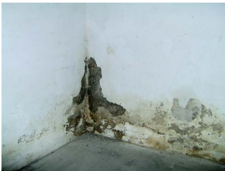
Dampness in Kiseljak Ammunition Depot building, which currently stores ammunition. Officers in charge pointed out that they needed materials to bring the buildings up to safety standards.
